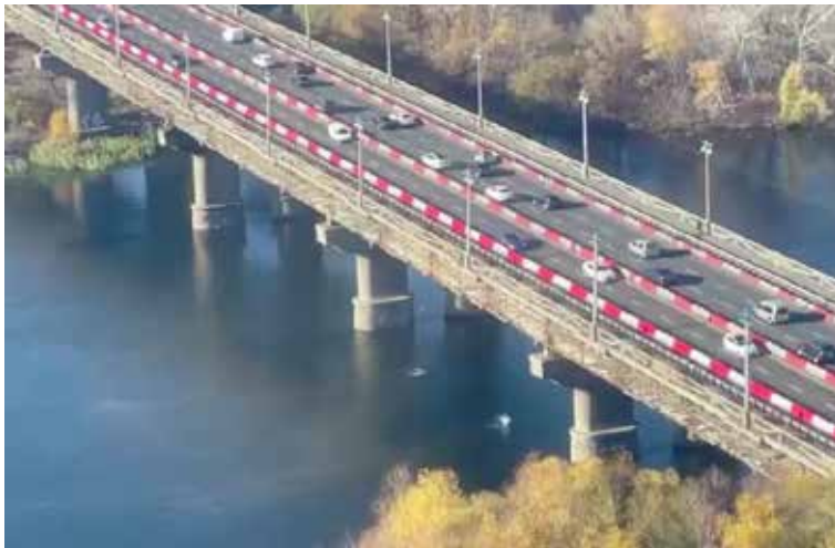
Fig. 1. Restriction of traffic on the two edge lanes of the Paton Bridge in Kyiv due to its poor technical condition
