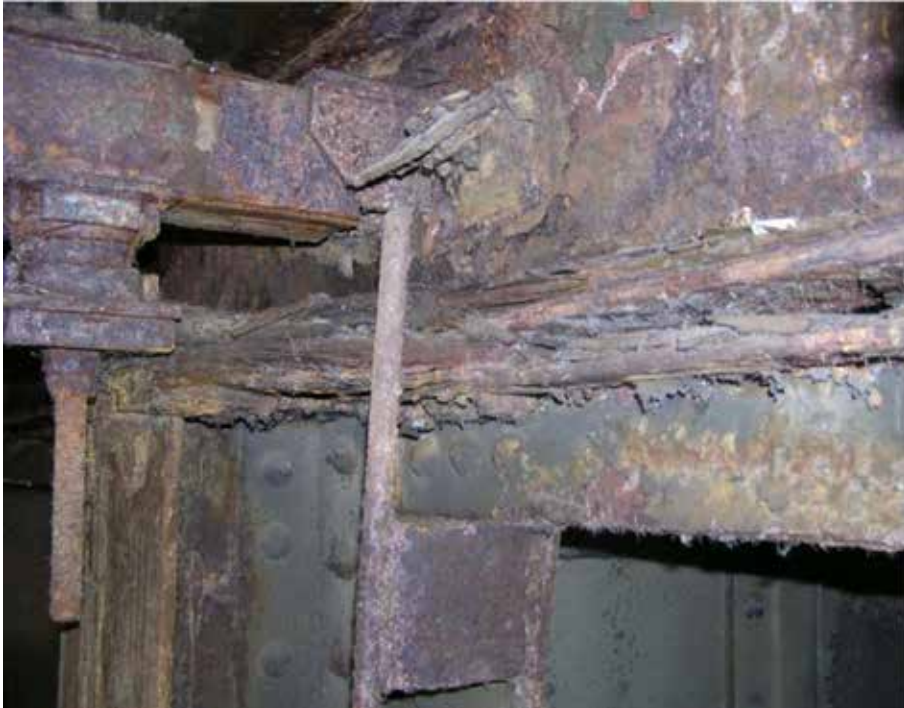
Fig. 2. Layering of the upper belt of the main beam of one of the transport facilities in Kyiv due to corrosion
